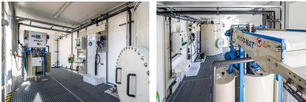
Image: View of the EnviModul with Split-O-Mat® SOM 500LB batch plant.
