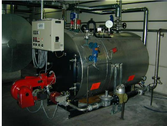
Figure 6: Steam boiler burning biogas
