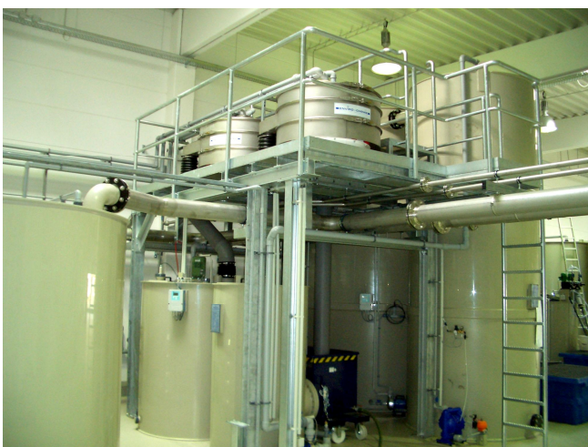
Fig-1: Example of a typical wastewater pretreatment stage (vibration screens, sand trap, etc.) of an Envopur UFI NA 2.000 ultrafiltration plant
