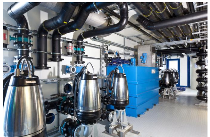
Part of an EnviModul wastewater treatment plant.
