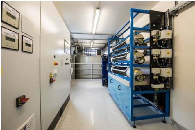
Image: Enviochem AOP plant installation; inside view of an EnviModul
