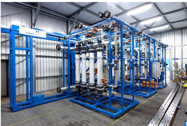
Image: EnviroChemie Envopur technology (view of the workshop)
